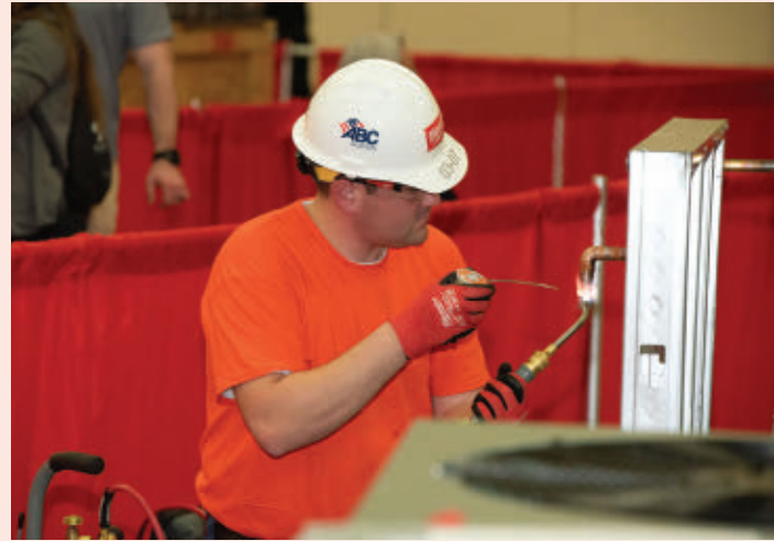
FIRE UP: Welding was among the 12 crafts represented at ABC's 2022 National Craft Championships.
